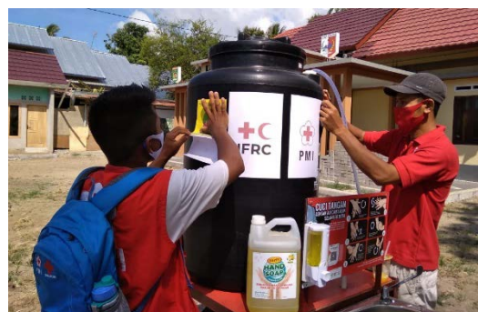
PMI personnel installing hand washing facility equipped with hand soap and IEC materials for handwashing tutorial in North Lombok. (Photo: PMI)
