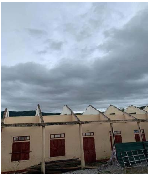
The roof of Quang Minh A primary school damaged by typhoon Vamco in Quang Minh commune, Ba Don town, Quang Binh province, 15 November. (Photo: VNRC Quang Binh Chapter)
