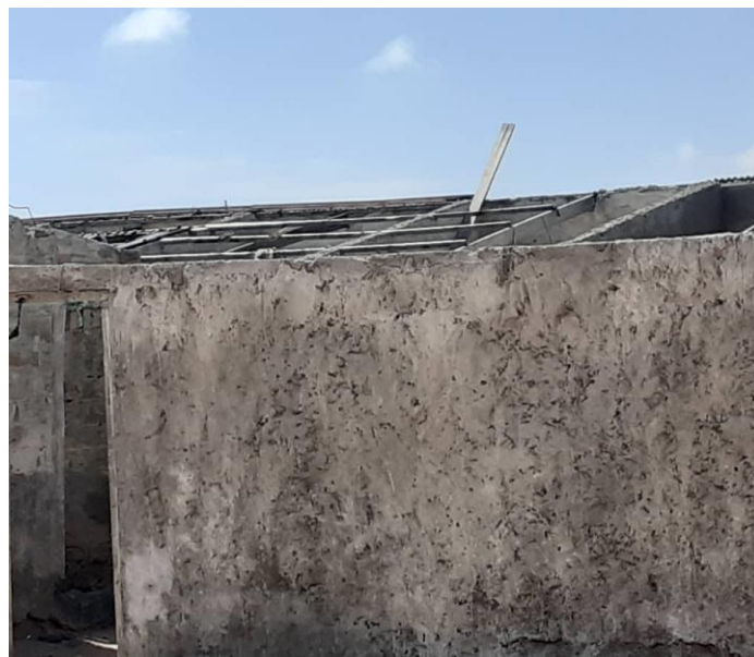
Roofs blown off houses as a result of TC GATO (Source: SRCS)
