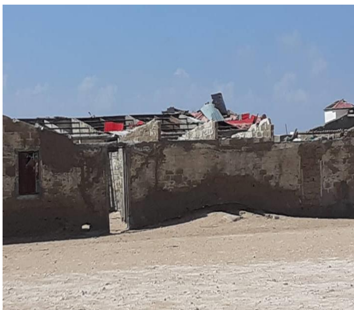
Makeshift repairs to homes in Hafun district (Source: SRCS)
