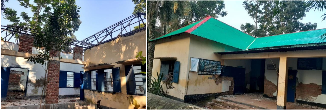
Ongoing repairing work in the Haidar Ali MCH Centre in Tangail. (Photo: BDRCS)
