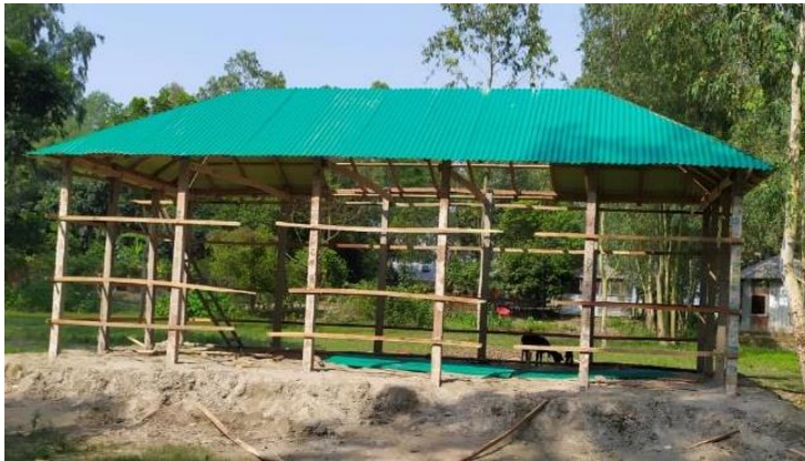
Through the owner driven approach, shelter construction is going on in Tangail district ( Photo: IFRC )
