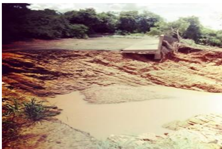
Kandesha Dam after the disaster ©ZRCs
