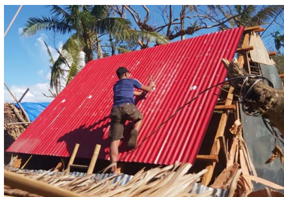
Fixing the roof with CGI sheets and tools provided by PRC (Photo: PRC).
