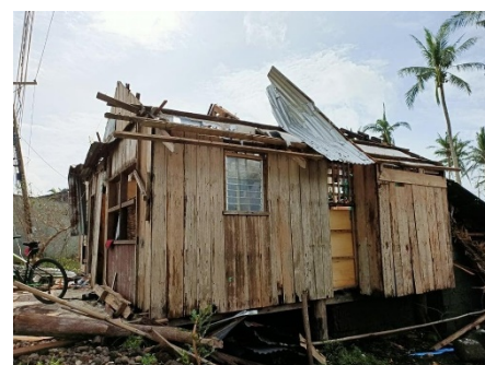
Super Typhoon Goni damaged many houses displacing families/people (Photo: PRC).
