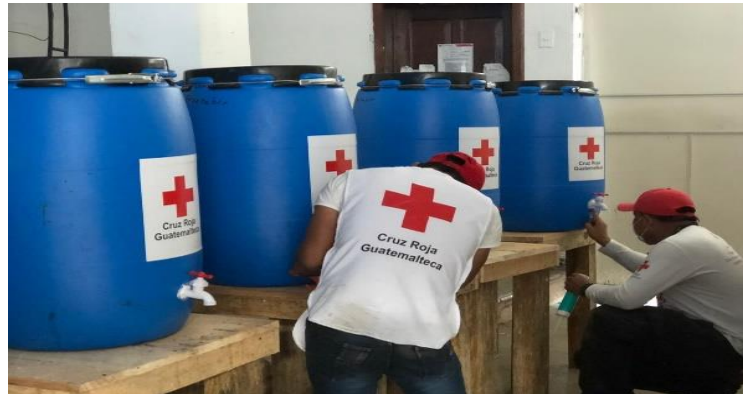
GRC team installing handwashing facilities in shelters in Campur. Source: GRC, December 2020.
