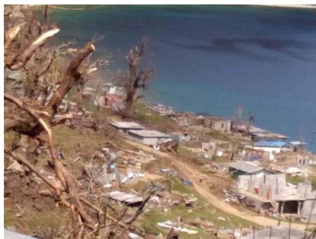
Damage caused by Category 5 Tropical Cyclone Harold at Mesis, Pentecost Island. Remaining as seen in the Photograph are Remaining of Foundations of Bank, Hospital school and sleeping houses of more than 1,305 families. (Photo: IFRC)
