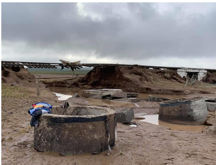
Railroad bed washed in Dornogovi province. (Photo: Eguur.mn)
