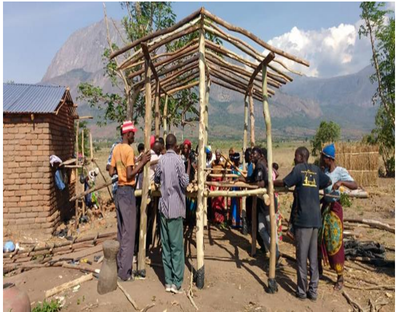
Beneficiaries in Mulanje District Constructing a Goat House. Picture by Malawi RC
