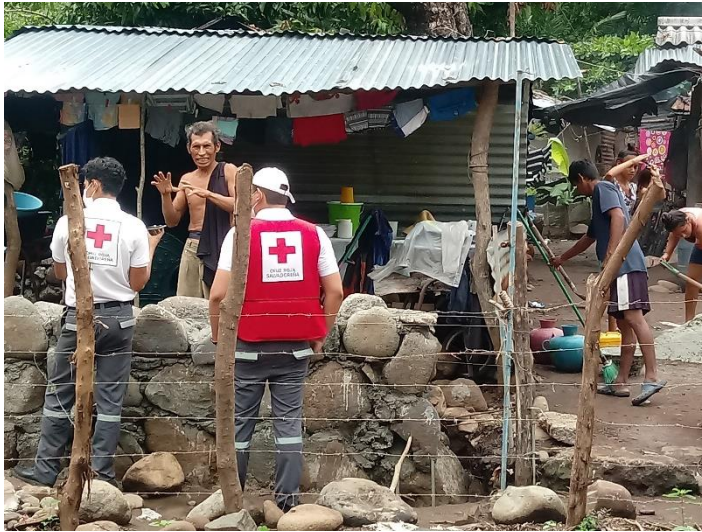
El Salvador RC team supporting the construction of a contingency wall at Mizata Community. Source: SRC
