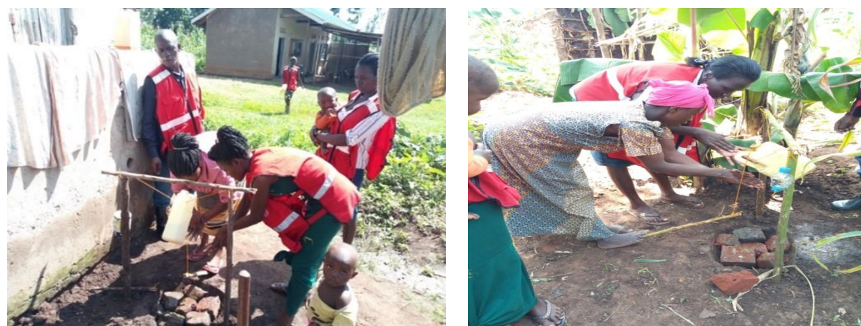
Figure 6: Volunteers construct tippy-taps demonstration stations to facilitate replication and improved hand-washing practices in Bududa and Namabasa, Mbale districts
