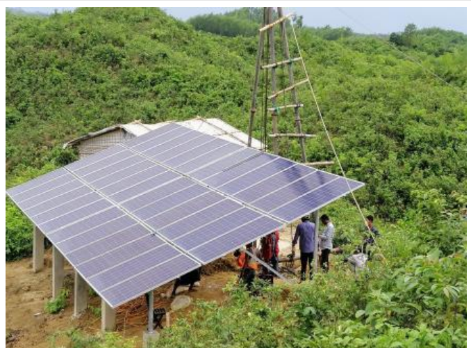
Camp communities are benefiting from an uninterrupted supply of safe drinking water thanks to solar-powered water supply systems established by BDRCS with IFRC support. (Photo: IFRC)
