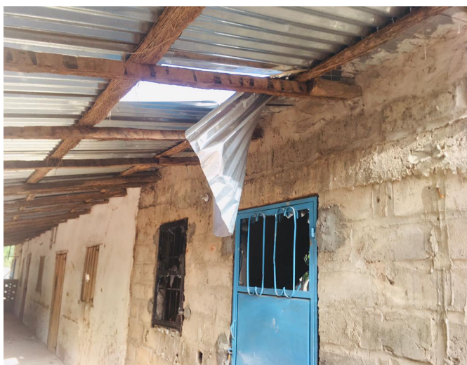
Damaged house resulting from communal violence in Sanyang Village ©GRCS
