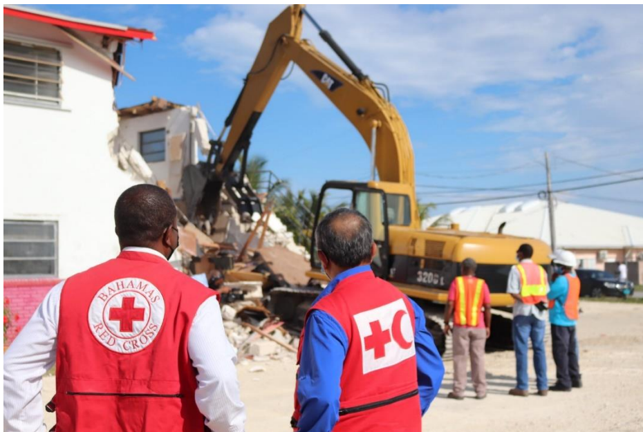
Demolition of the BRCS Grand Bahama branch building was completed in January 2021 (Photo: BRCS)
