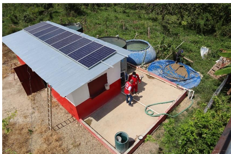
PRCS volunteers work on the water purification facility in Darien in January 2021. Source: IFRC
