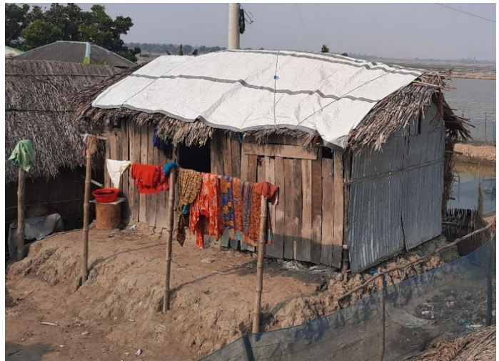
One of the affected households using the tarpaulin that received from BDRCS on the roof in Khulna. (Photo: IFRC)
