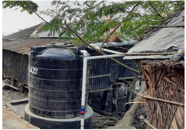
One of the newly installed rainwater harvesting systems in Khulna district. (Photo: IFRC)
