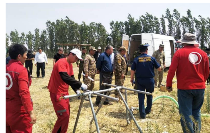
Picture 6: Installation of water tank in cross border Maksat village. Photo credit: RCSK
