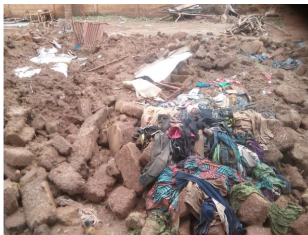
This is what remained from a house after the passage of the flooding in Kaya @ BRCS
