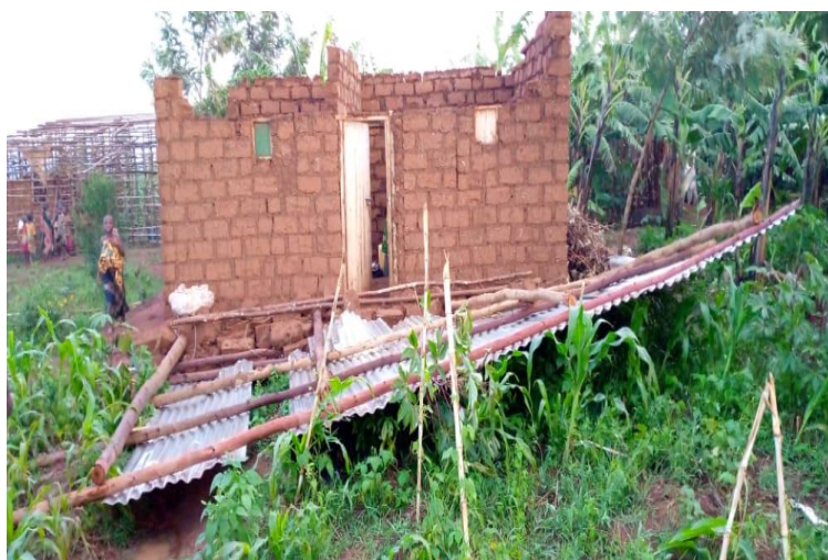
Damaged house in Kayonza ©RRCS
