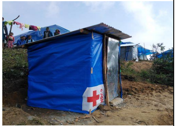
A temporary toilet constructed with the support from NRCS at a temporary shelter in Sindhupalchok district. (Photo: NRCS DC)
