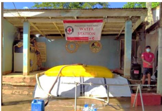
Fully installed 5,000 liters water bladder with tap stand in Cagayan. (Photo: PRC)
