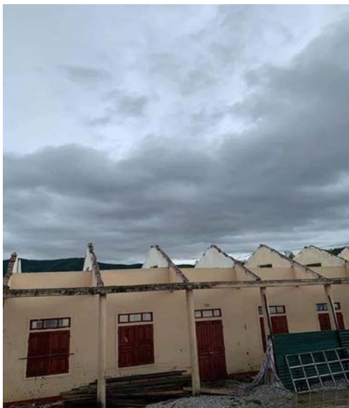
The roof of Quang Minh A primary school damaged by Typhoon Vamco in Quang Minh commune, Ba Don town, Quang Binh province, 15 November. (Photo: VNRC Quang Binh Chapter)
