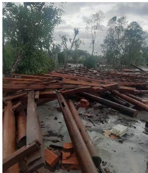
House totally collapsed in Quang Long district, Quang Binh province, 15 November. (Photo: VNRC Quang Binh Chapter)
