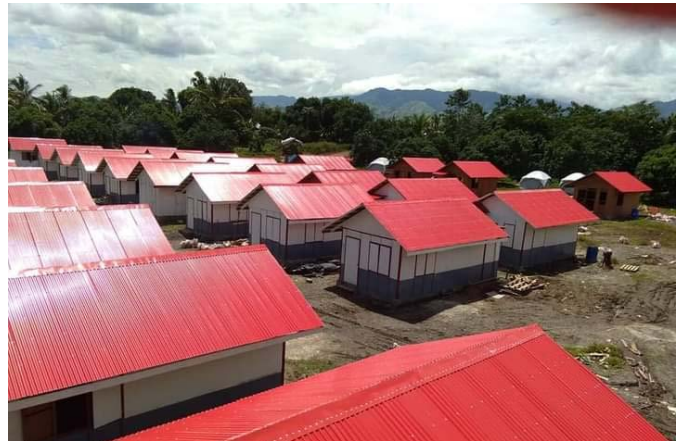
In collaboration with the local government unit, PRC was able to construction shelters for the most vulnerable displaced families affected by the earthquake. (Photo: IFRC)
