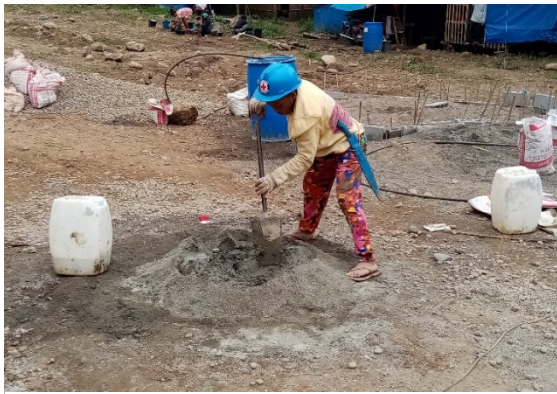
Participation of women played a critical role in the implementation of the shelter project in Mindanao earthquake response, (Photo: IFRC)
