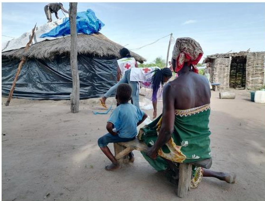
1 / 2 Red Cross volunteers assist vulnerable households in the reinforcement of their houses (Source: Mozambique Red Cross Society)
