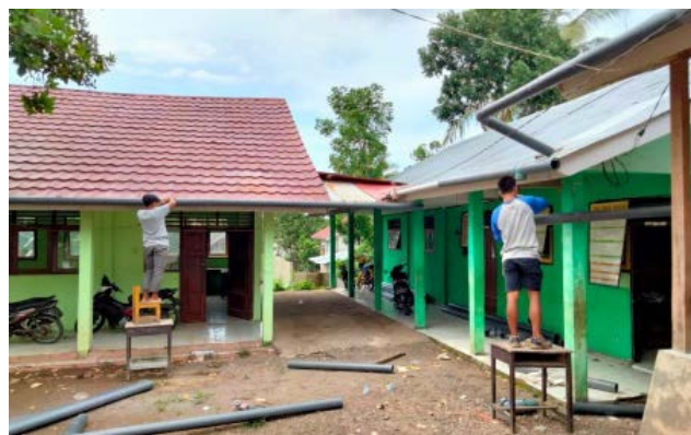
Instalment of gutters to convey water from the roof to water storage Photo: PMI
