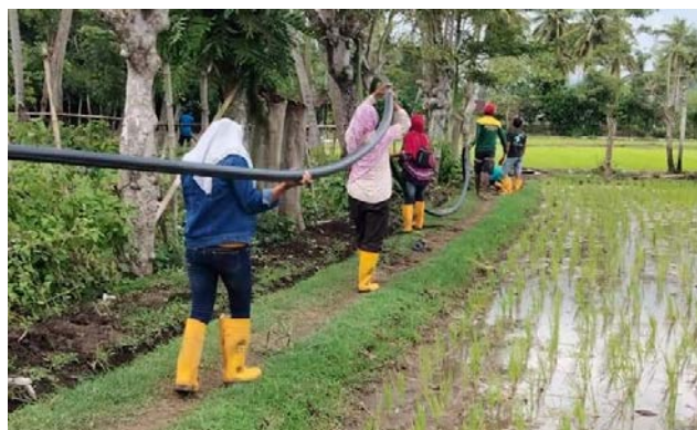
Pipeline installation in Lamunga village to deliver water from water spring to the community. Photo: PMI
