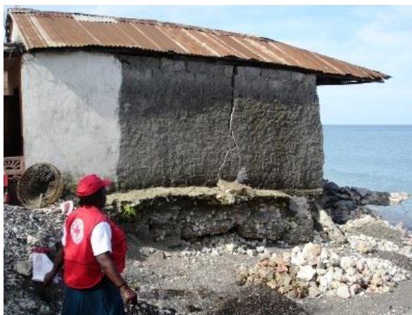
One of the damaged houses in Dame Marie. Impact assessments from the Government of Haiti indicated that 24,348 houses were damaged. 2012. Photo: IFRC
