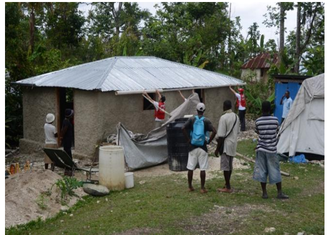
CTU Gond-Ayer nearing completion. MSM-ERU worked together with HRCS to improve a total of 19 CTCs/CTU according to the identified needs from the assessments. Photo:IFRC
