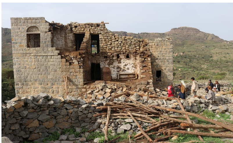
Figure 1: Damages caused by heavy rains in Al Mahwit governorate. YRCS staff and volunteers were deployed in Al Mahwit and other governorates similarly affected by the ongoing rainy season and subsequent floods to provide immediate assistance such as early warning, search and rescue, first aid and emergency relief through the distribution of food and non-food items including hygiene kits, as needed. Photo: YRCS
