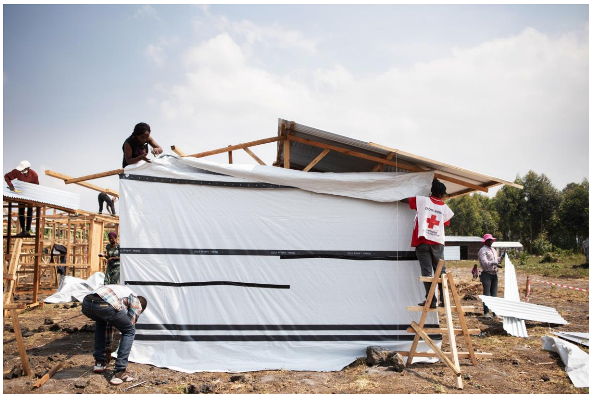
Shelter construction by DRC volunteers at temporary relocation site in Kibati, DRC. © IFRC
