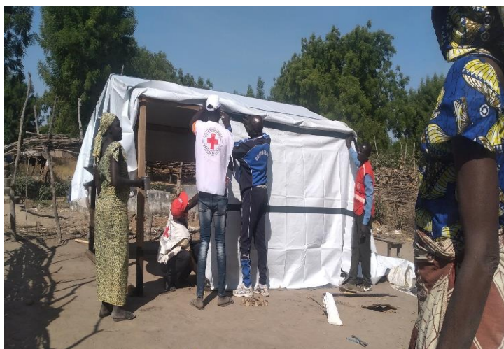
Construction of a shelter with the help of CRC volunteers. Credit: CRC
