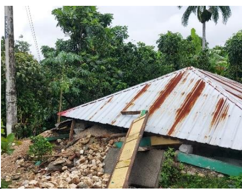
Home destroyed by the earthquake in Torbeck, Sud department. Source: IFRC Relief ERU.
