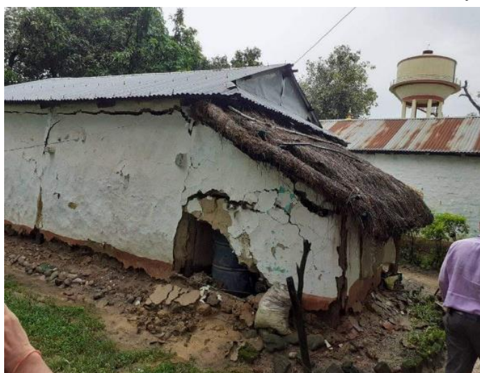
A house damaged due to the intense rainfall in Rupandehi district. (Photo: NRCs)
