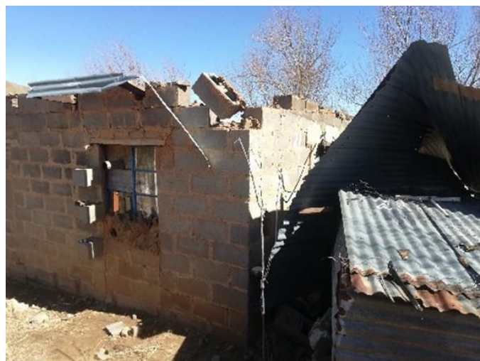
Damaged house in Qacha's Nek ©LRCS
