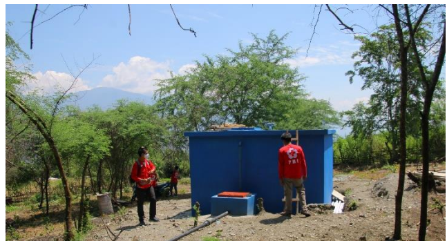
Gravitational water supply and reservoir in Sibowi village.
