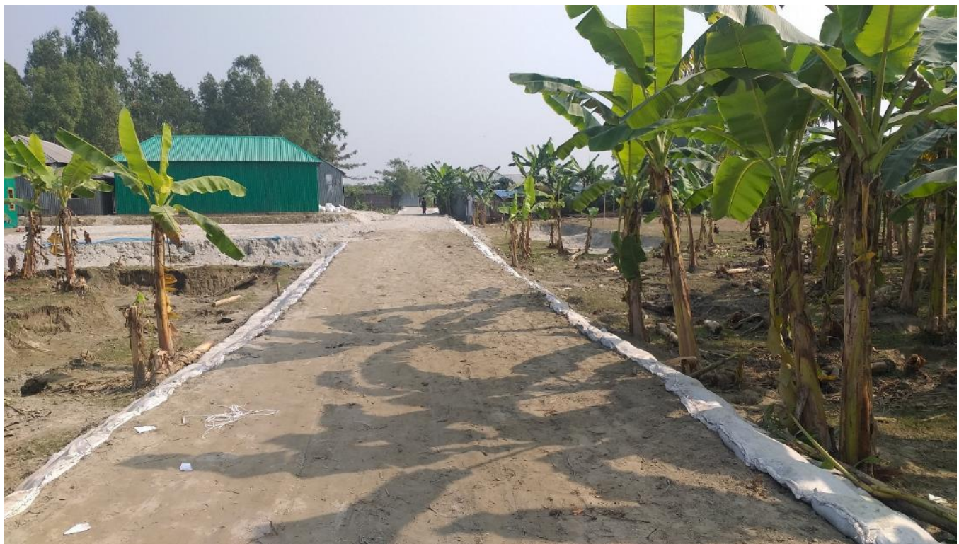
1,420 feet earthen road constructed in Tangail under Cash for Work as a part of the DRR. (Photo: BDRCS/IFRC)
