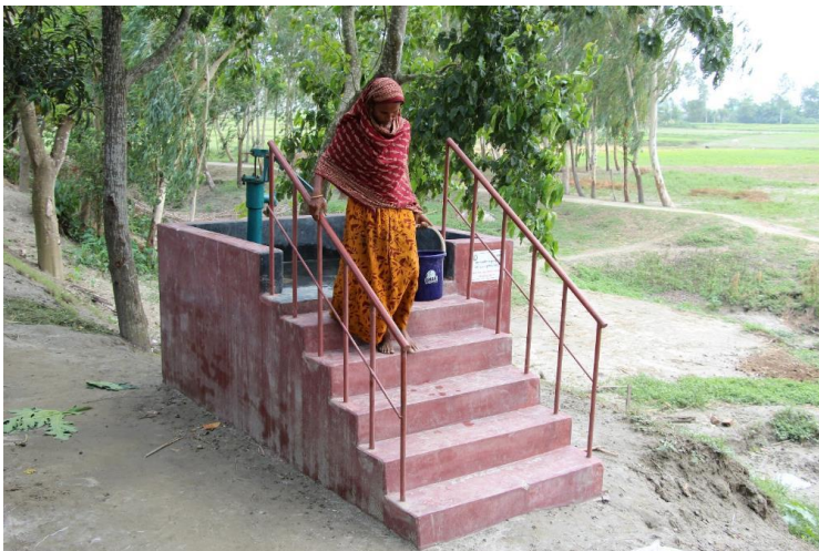
Flood resilient tube wells have installed in the community, which will meet the water needs of the community during floods. (Photo: BDRCS/IFRC)
