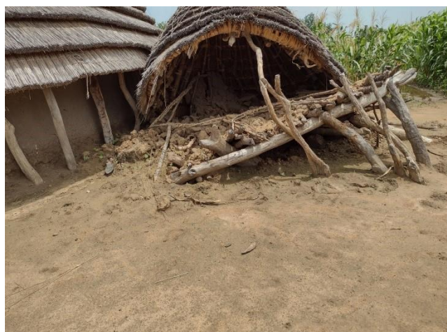
Floods destroyed house in Langthok Village, Gogrial West County ©Inter-Agency Needs Assessment Team, July 2021
