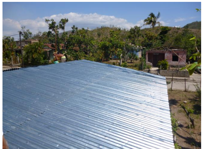
One of the first repaired in a house in a community in the province of Santiago roof de Cuba. Source: Cuban Red Cross
