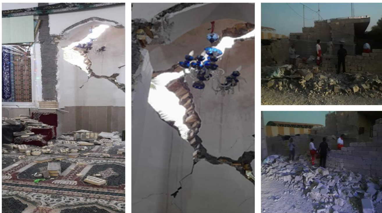
Figure 1: Structural damages caused by the earthquake. Credit: IRCS
