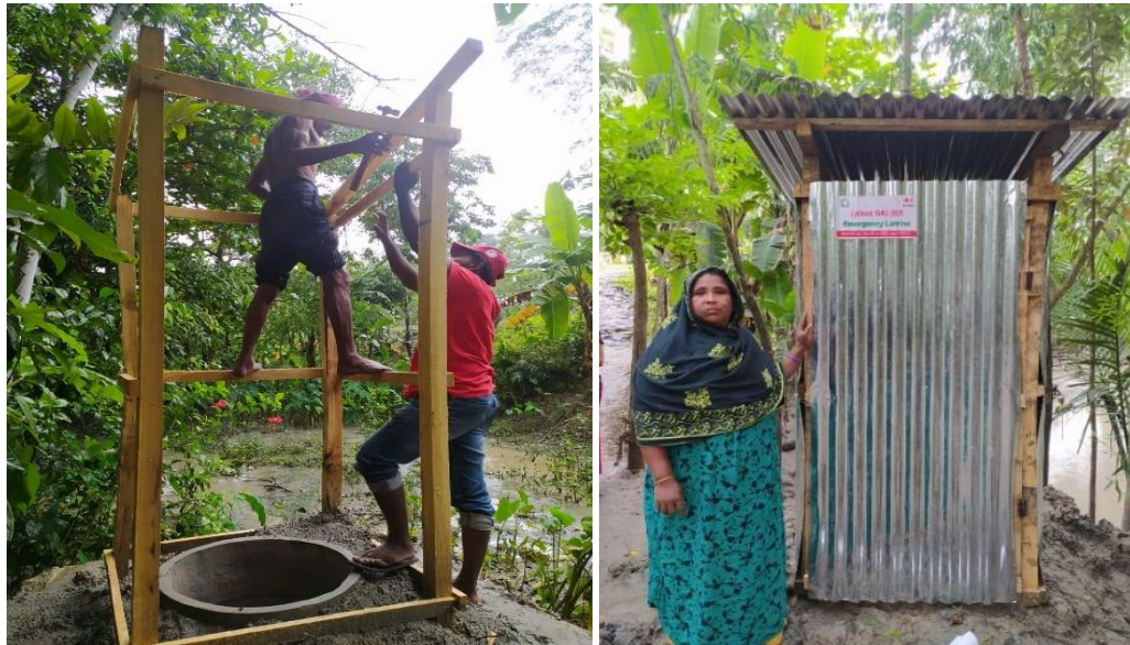
Construction of a communal latrine (L); An owner standing by her newly installed latrine (R) (Photos: BDRCS)
