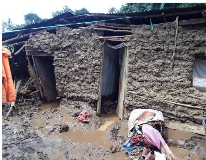
Damaged House in Mbeya region ©TRCS
