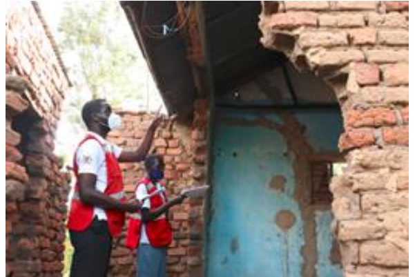
Damaged house in Mbale district ©URCS
