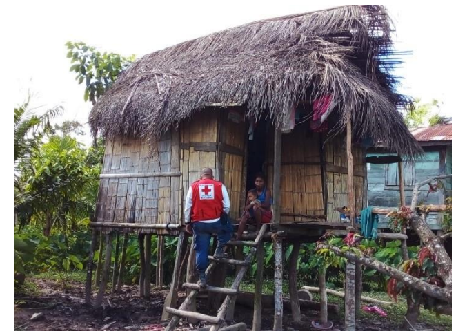
Identification of inadequate housing, Waspsam, November 2021 Source: NRC
