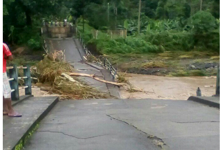
The bridge over the Lemba River collapsed due to heavy rains in Sao Tome and Principe on 28 December 2021 © CONPREC
