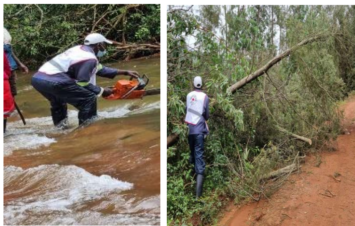
Figure 1: ZRCS volunteers assisting clearing roads blocked by trees felled by TD Anna induced strong winds and rain. ©ZRCS
