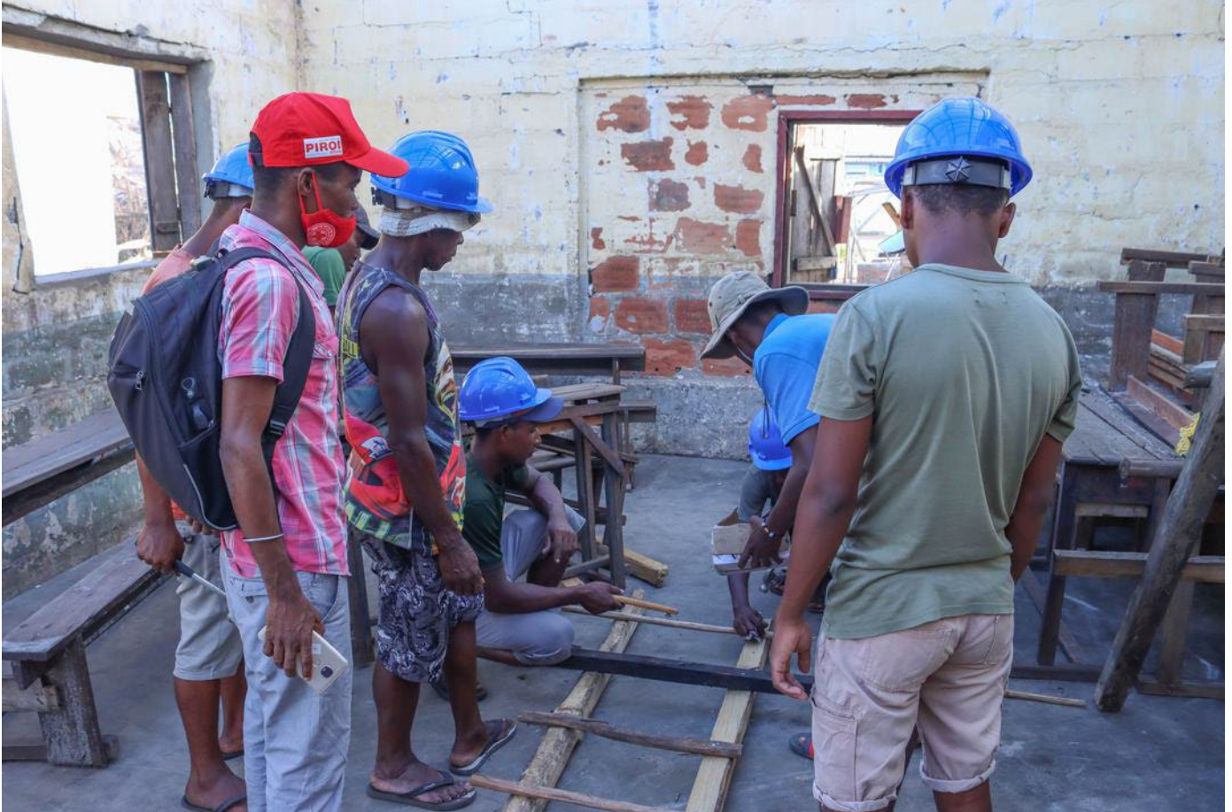
Figure 1: Skilled workers supervised by Red Cross team member while they work on improving a spontaneous shelter ©IFRC
