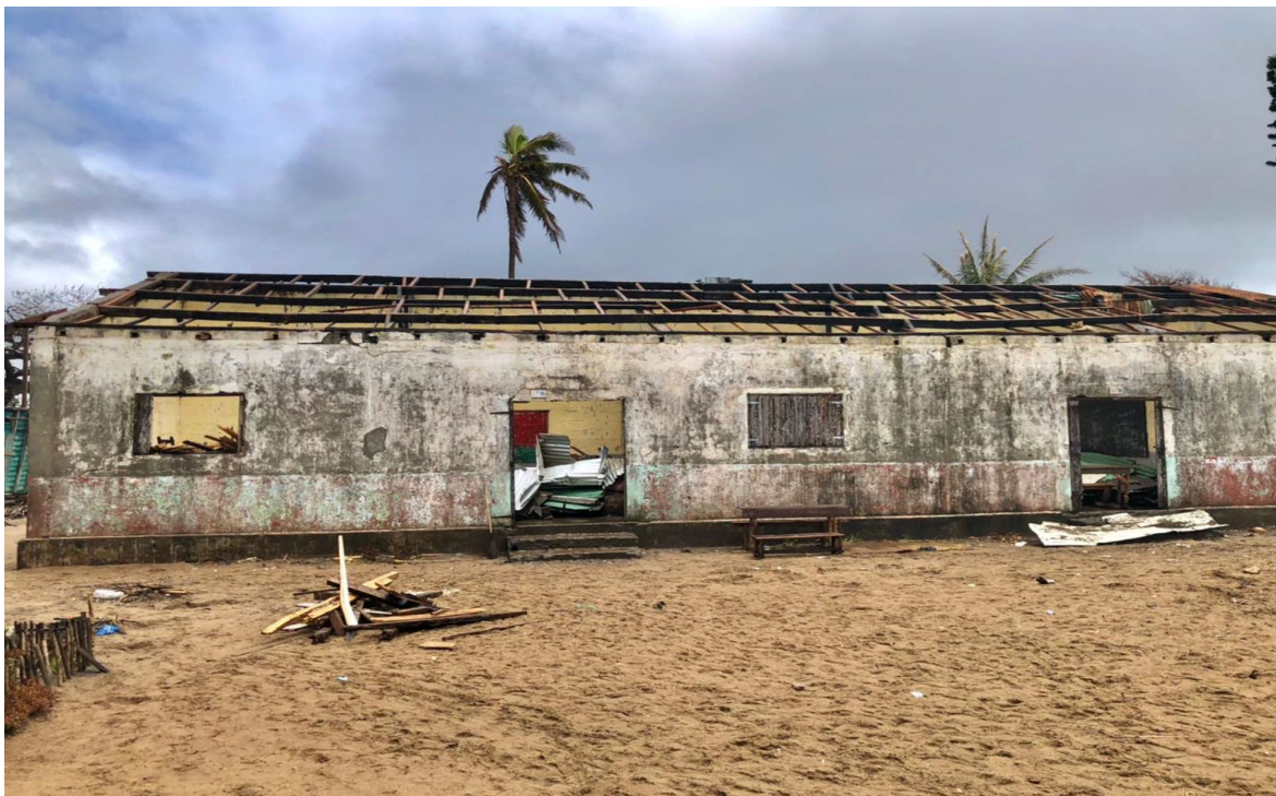
Figure 2: Roof of the Public Primary School “EPP” Masindrano blown away, although families still hosted ©MRCS/IFRC
