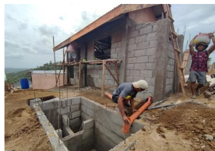
Construction of septic tank of the latrine, which is intergral component of full shelter assistance. Photo: PRC
