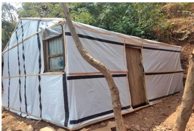
Sample of an emergency shelter constructed by BRCS for floods affected households ©BRCS
