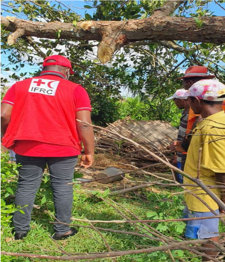
IFRC inspect latrine of a household that has been damaged as a result of TC Batsirai during a rapid assessment in Sandrohy commune (Photo © IFRC)
