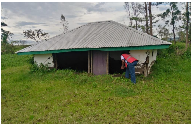
Figure 8: Ongoing assessment in West Kenya Region- Abandoned houses
