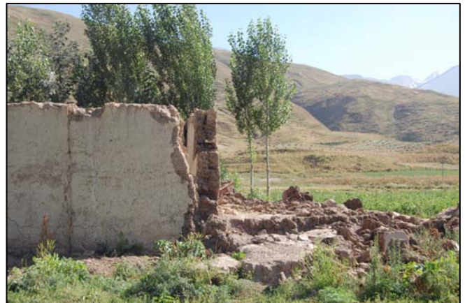
Building destroyed by an earthquake in Rasht region. Photo: IFRC
